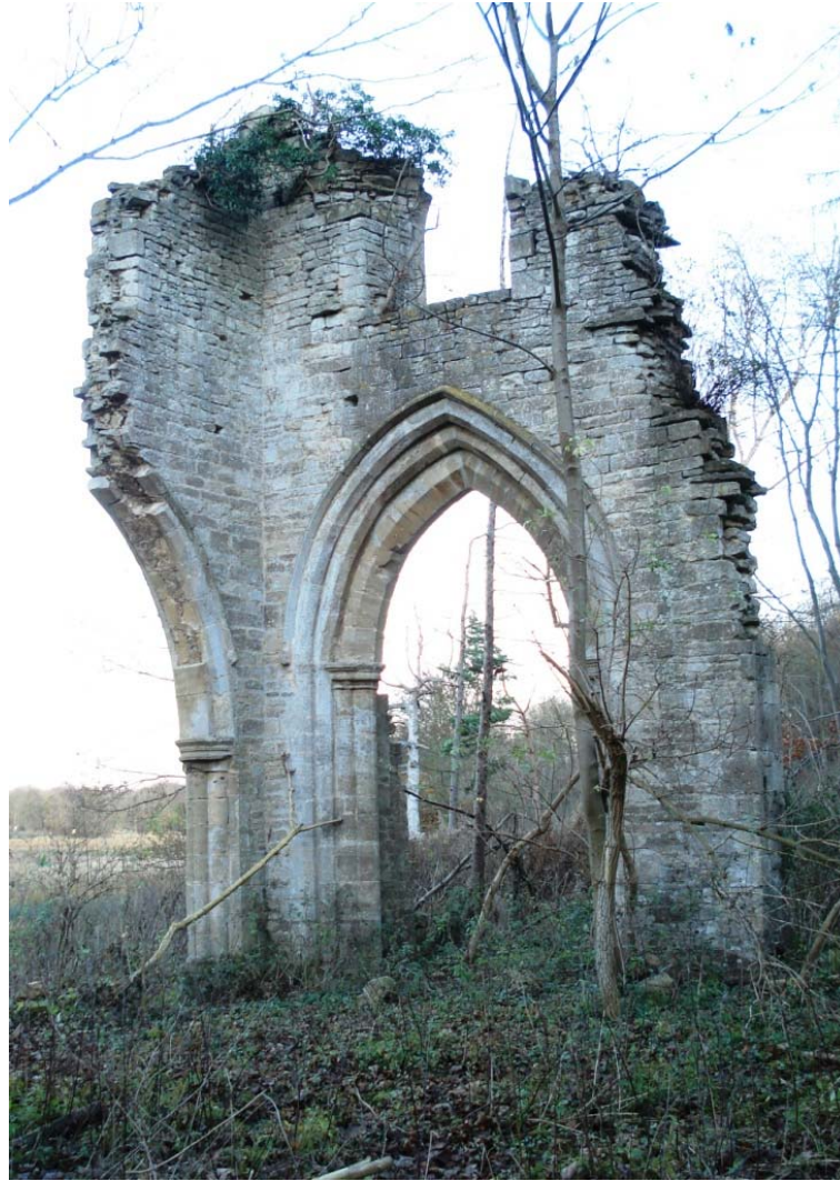
Figure 3: The remains of St Peter's church Lilford, rebuilt as folly near Achurch.
